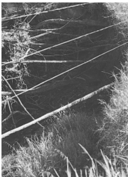
Plate 10: Close up of fence-line and subsidence.
