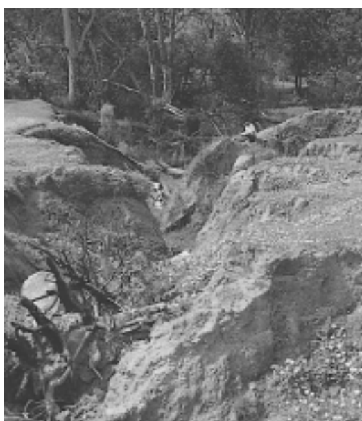
Plate 12: Severe gully erosion on the Capel River.
